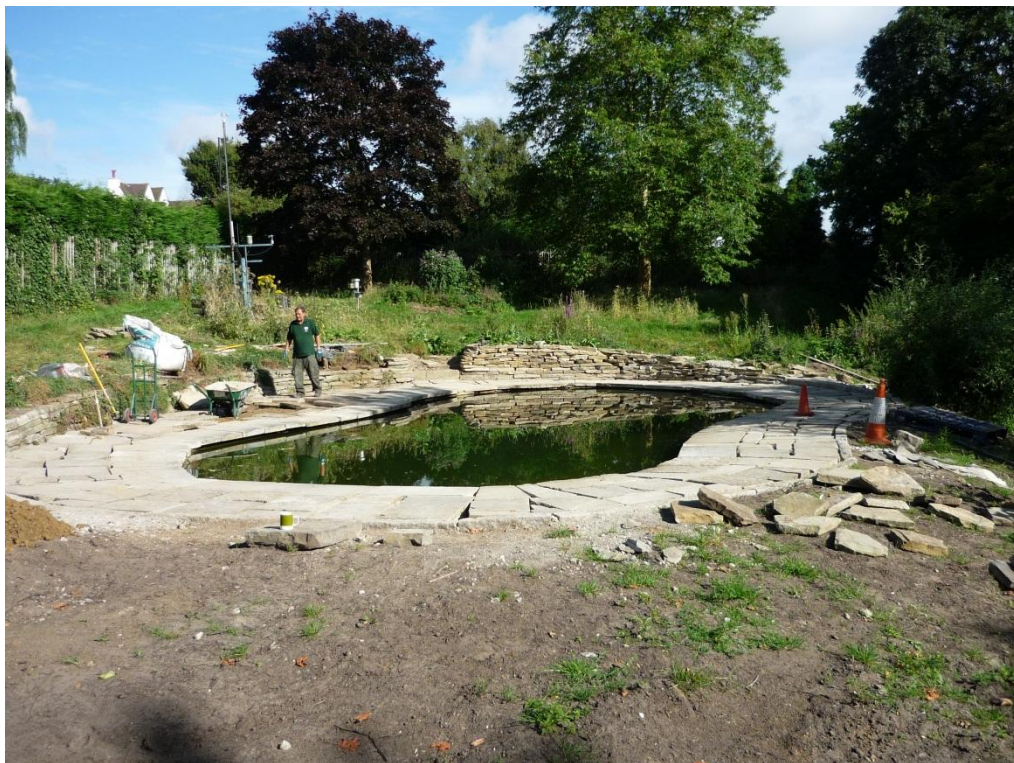
Figure 1: New pond under construction at Kenwood Nursery Yard as part of CBT project
